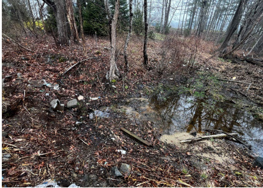
Photograph 8a: Looking east, storm drain pipe to left of rock underneath green ash tree, pipe above highest observable tide line; April 2024
